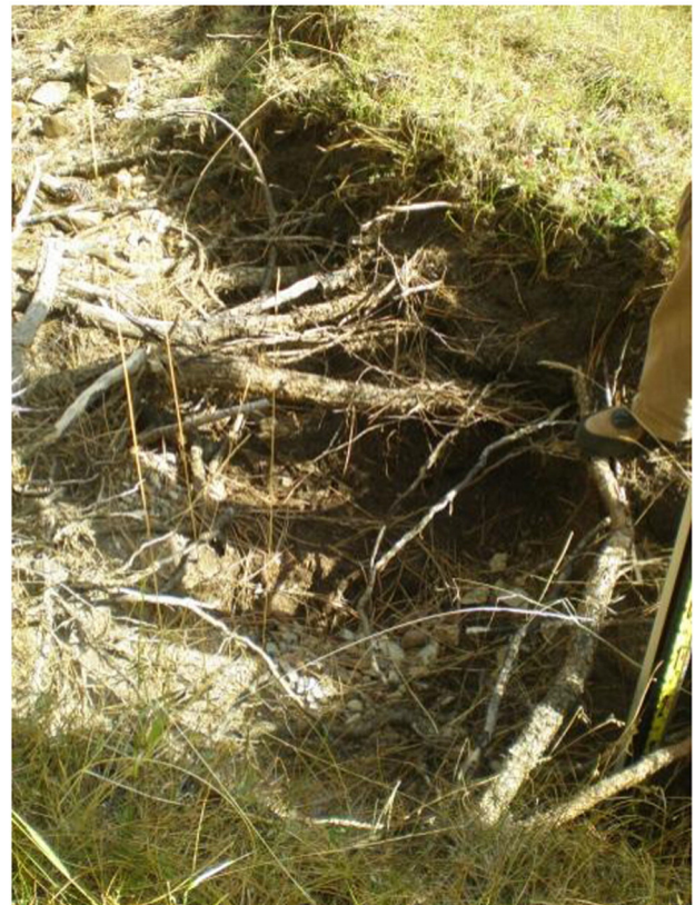
Fig. 10. A scour pool caused by extensive tree roots in Carman Creek, Three Corner Meadow.
