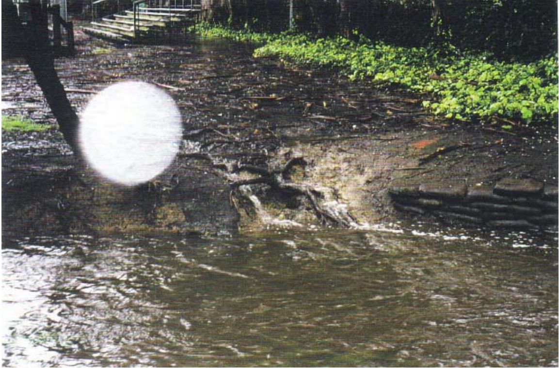
Figure 46: The downstream end of Baxter Creek in Booker T. Anderson Park showing the gully being created, as well as the banks bolstered with “sack-crete.”
