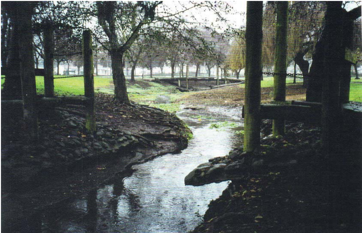
Figure 22: The remnants of an old bridge show how the creek has eroded its banks beneath the bridge footings (top); on one bank, a gully has been created by a pipe directing subsurface flows into the creek (bottom). Photos by author. 2000.
