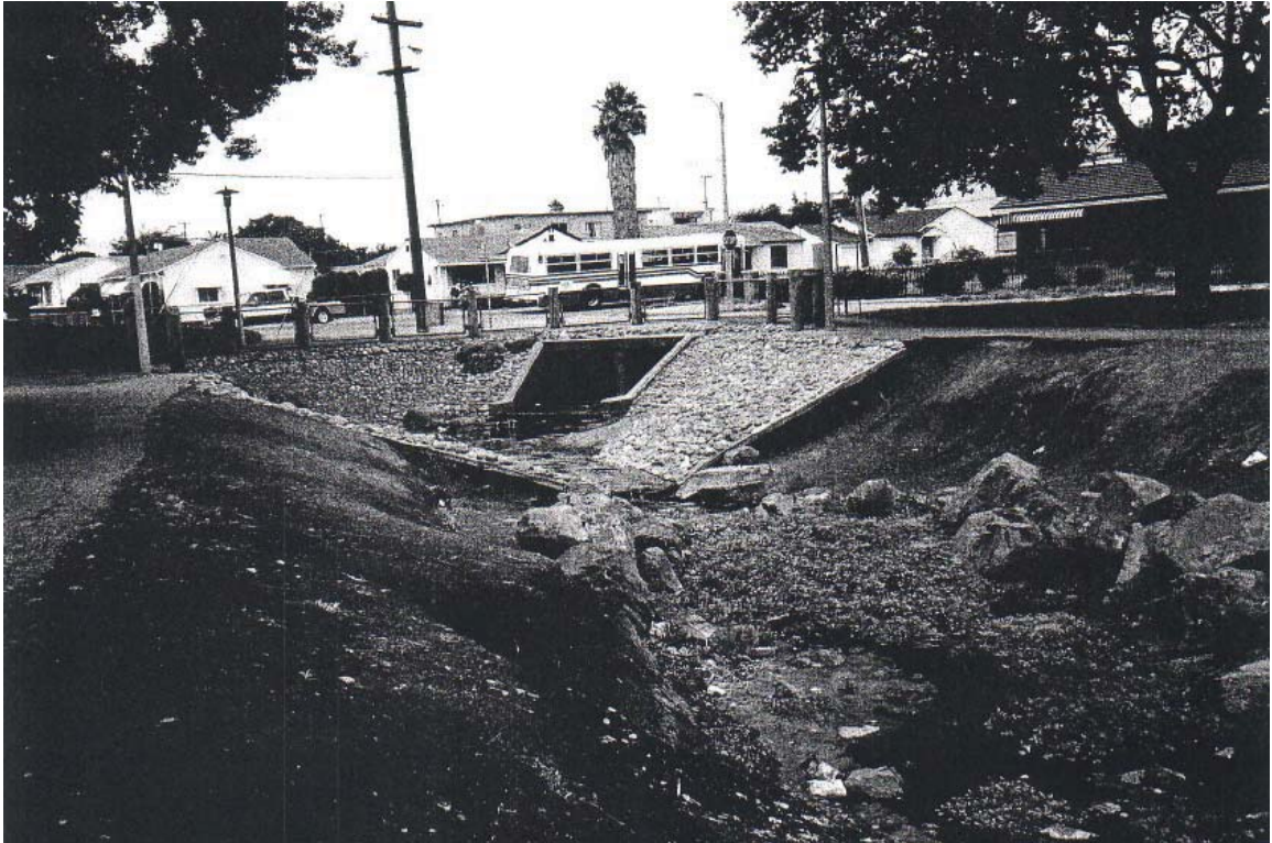
Figure 21: Unsuccessful and unattractive engineering: cobble rockwork at mouth of culvert entrance, Booker T. Anderson Park—note erosion beneath the cement. Large boulders placed on the creek's banks washed or have fallen into the creek bed. Photos by author. 1999.
